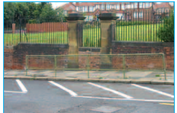
This guardrail has no function - the pedestrian route it was protecting has been closed - and can therefore be removed.
