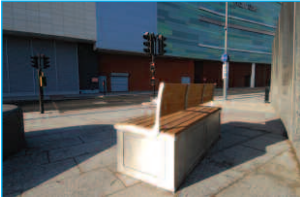
Bench containing traffic signal controller
